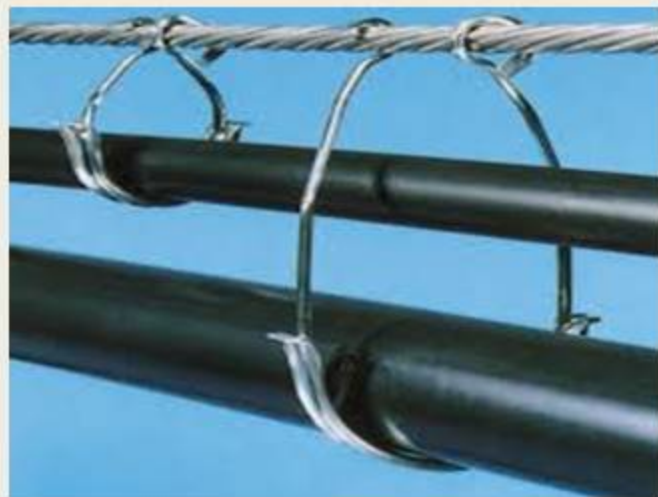
Aerial cable on a messenger
