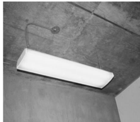
PHOTO 20.20 A linear fluorescent luminaire with prismatic wraparound lens that diffuses light. (Used with permission of ABC)
