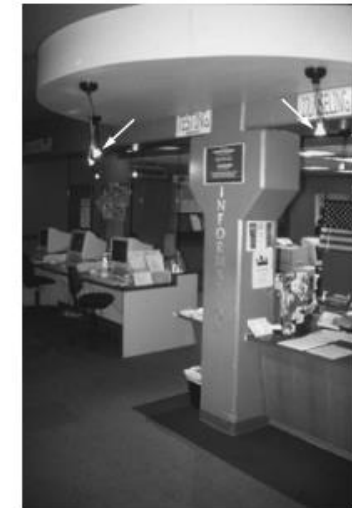
PHOTO 20.30 Decorative halogen accent lighting can add interest to a space but can also cause glare. These eye-level accent lights were intended to provide accent and task lighting, but they adversely affect visual comfort from glare at eye level. (Used with permission of ABC)
