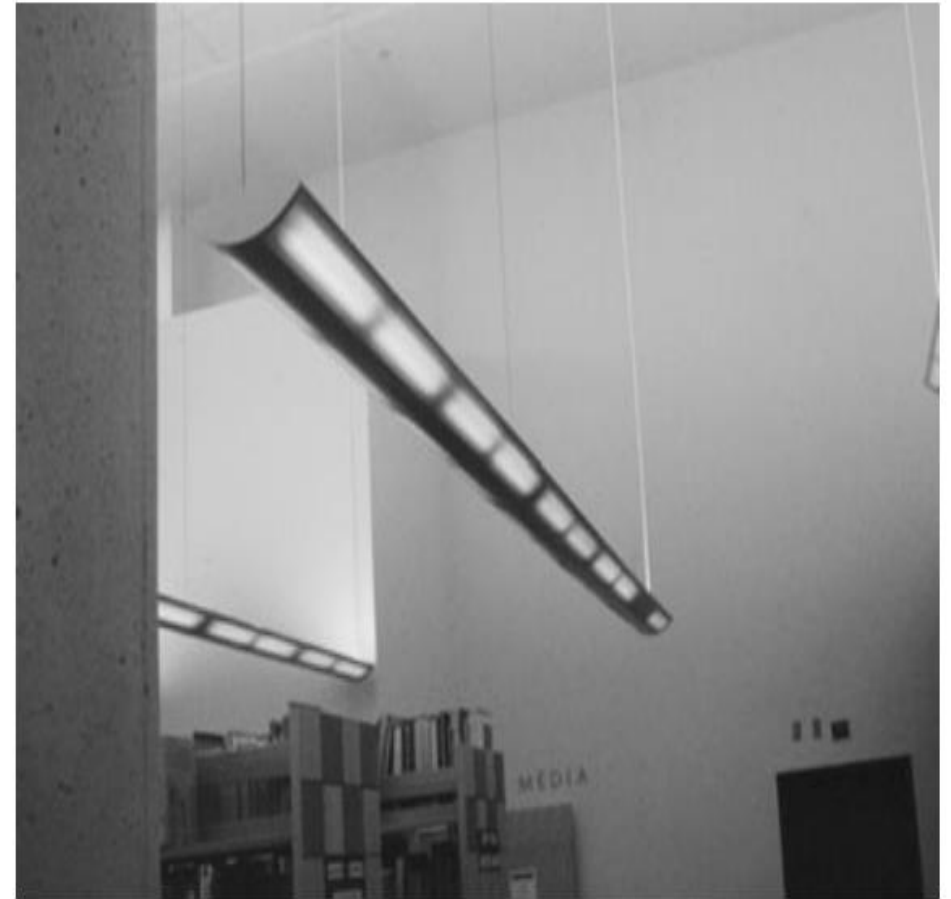
PHOTO 20.9 A linear fluorescent uplight used to provide ambient lighting in a library. (Used with permission of ABC)
