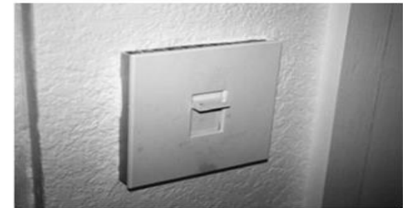
PHOTO 20.32 A wall-mounted dimmer switch used to control several banks of track lights.
