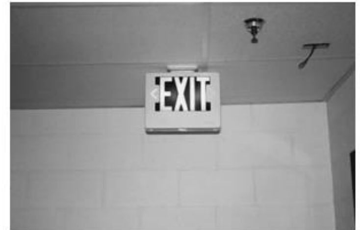
PHOTO 20.31 Exit lighting. (Used with permission of ABC)
