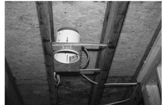
PHOTO 20.13 A recessed light fixture during construction. After it is secured to the joists, placement of the fixture can be adjusted (left to right). (Used with permission of ABC)
