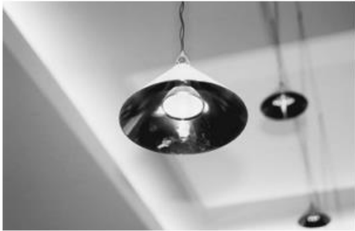
PHOTO 20.29 Halogen accent lighting used as task lighting over a conference table. (Used with permission of ABC)
