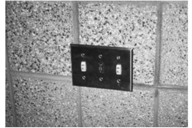
PHOTO 20.33 Ganged (multiple) key switched.
