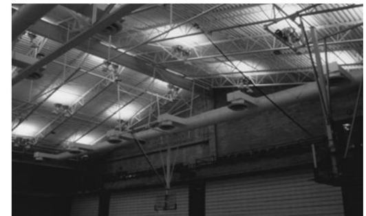
PHOTO 20.11 An HID uplight installation providing ambient lighting in a gymnasium. (Used with permission of ABC)
